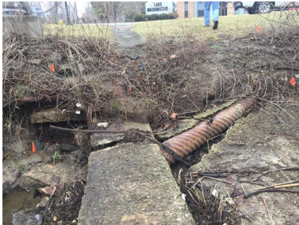
Storm Infrastructure Issues
