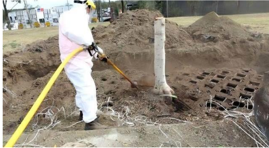
Figure 15 - with the Root Grid membrane and ReRoot linear barrier removed, air excavation commenced to start to unveil root growth.
