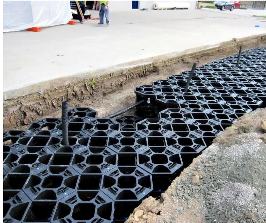
Figure 9 shows the initial Stratacell layers being installed in 2011. Note the depth of concrete on one side, and RootRain piping incorporated into the Stratacells.
