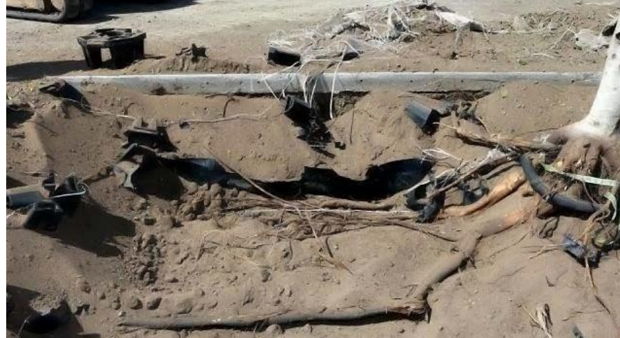
Figure 19 - excavation by air and machine expose roots that have descended to a depth of 700 mm then spread through the Stratacell voids in a linear fashion.
