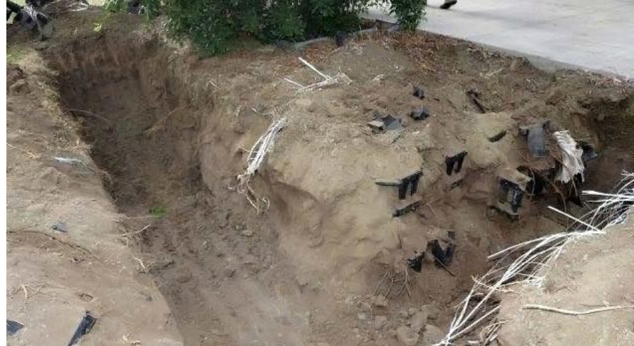
Figure 11 shows the view looking at the trenches excavated about Tree 1 with some of the exposed Stratacells and Root Grid.
