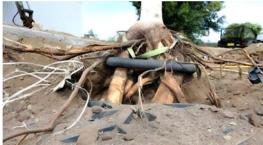
Figure 18 clearly shows the downward initial root growth caused by ReRoot linear barrier. The Root-Rain Piping and security straps did their job. The diameter and number of roots present was observed as well as the deep penetration of roots.
