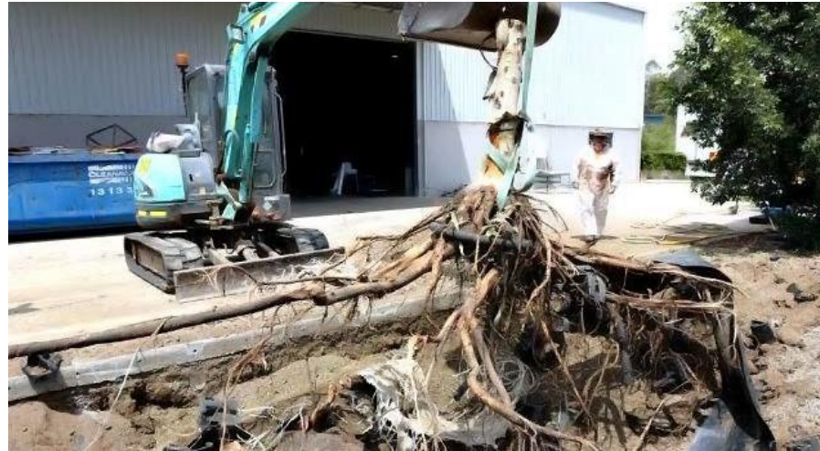
Figure 21 - after considerable mechanical excavation occurred, the final root system was removed, complete with root barrier, sections of RootRain and Stratacells where roots had grown well through the layers.
