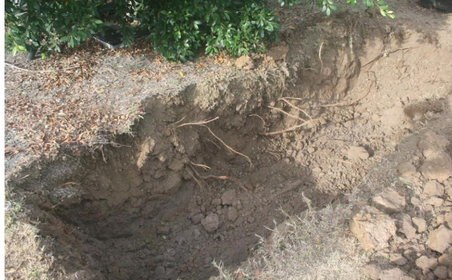
Figure 3 shows the first trench excavated, exposing the edge of the tree vault system. The trench edge was 1.6 metres from the trunk on this side. Note the presence of roots (15 – 25 mm diameter) found at the edge of the vault.
