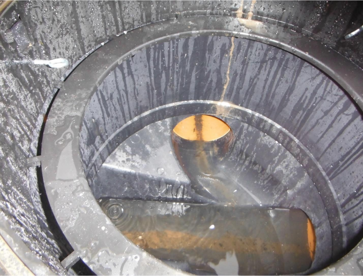
DSCF0323 - Water flowing into the system from parking lot strip drain.
