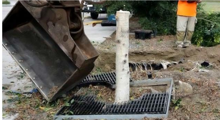
Figure 13 - the canopy has been removed and the excavator dismantles the tree grate system. The RootRain piping is partially exposed.
