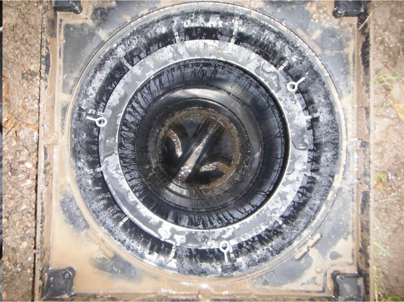
DSCF0319 - shows outlet drain - no water flow outwards after 2 hours of rain fall, demonstrating attenuation in action. Some post installation debris visible. This is 80" (2m) down.
