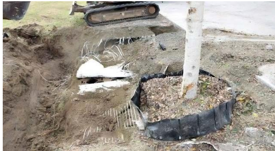
Figure 14 - using the excavator to remove the uppermost layer of gravel and expose the Ribbed linear root barrier.
