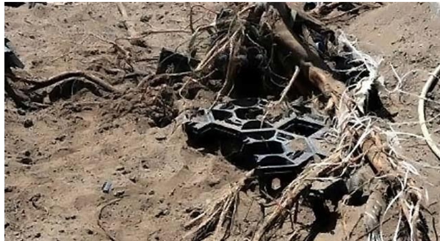
Figure 20 - this image shows how the roots grew in several directions. The majority of root development was parallel to the edge of the concrete. Large roots were present just above the RootRain pipes. Other roots grew at 90 degrees to the root barriers and concrete edge. Most lateral spreading roots were present at a depth of 600 – 700 mm or lower.
