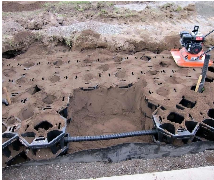
Figure 10 shows the backfilling of the Stratacells with sandy loam growing media and compaction. A root barrier has been placed between the Stratacells and the concrete forecourt with a strip of fine gravel approximately 250 mm wide placed against the concrete to minimize root invasion. The planting hole is prepared and ready for completion.
