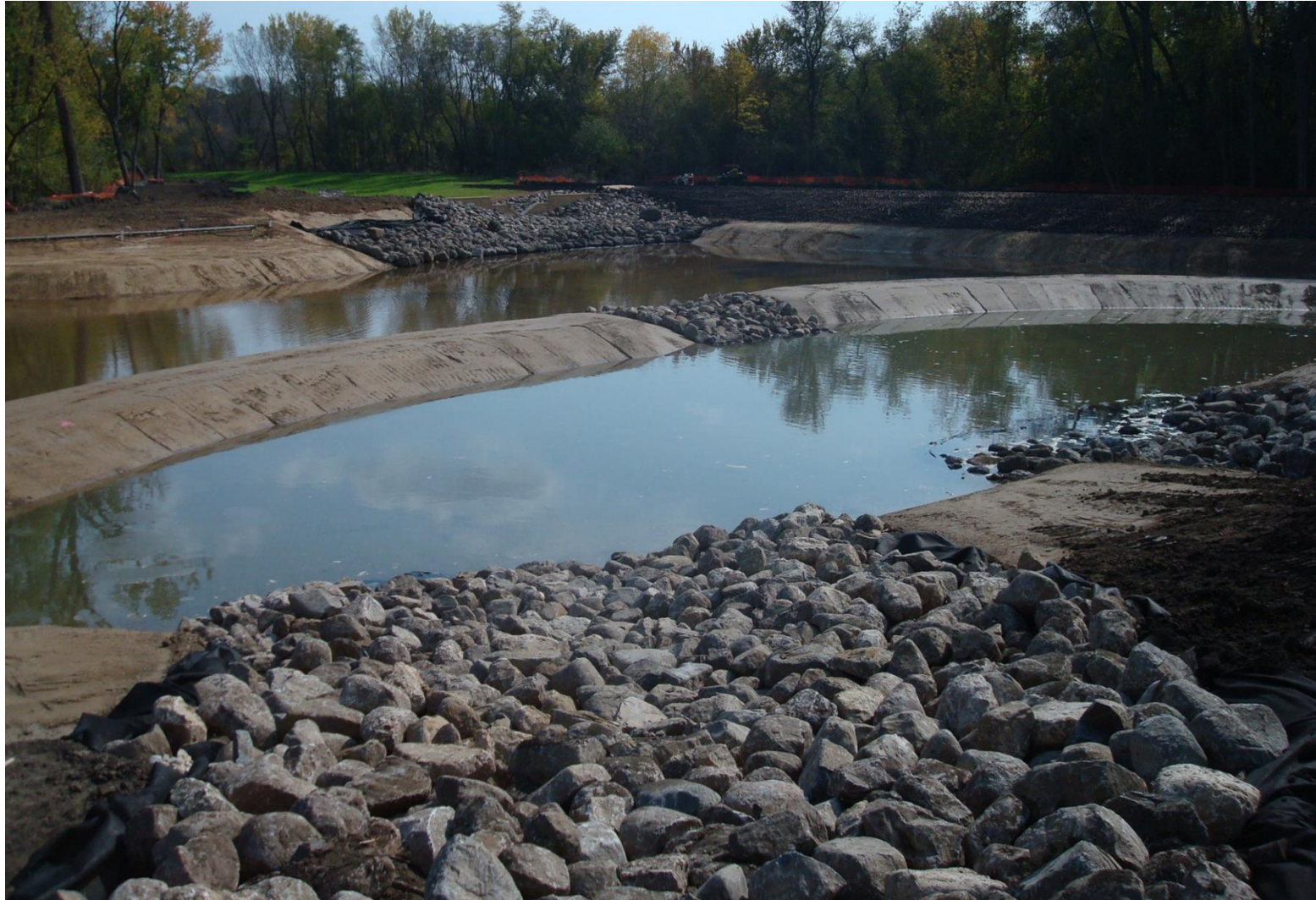
Pond partially filled with water prior to a large rain event that filled the pond completely.
