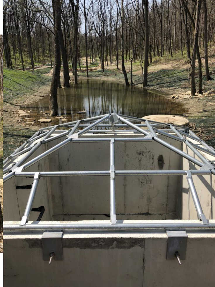
Detention Outlet Control Structure
